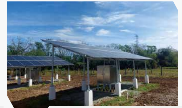
Six 10kVA photovoltaic energy storage systems in the Philippines
