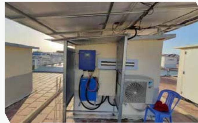
Cambodia 5kVA photovoltaic off-grid system
