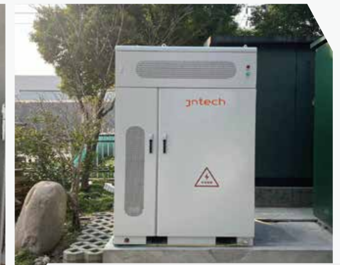
Hefei 100kW/200kWh energy storage system
