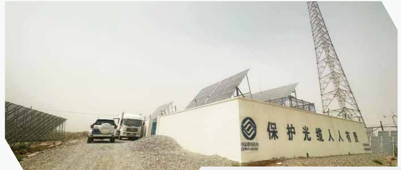
Xinjiang Korla region China Mobile base station project
