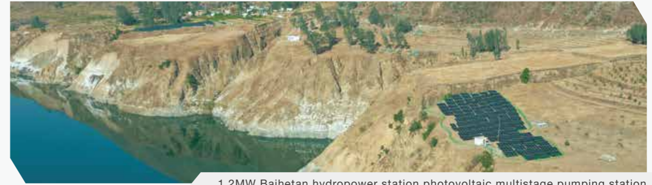
1.2MW Baihetan hydropower station photovoltaic multistage pumping station
