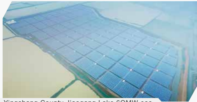
Yingshang County Jiaogang Lake 60MW ecological agriculture photovoltaic power generation project
