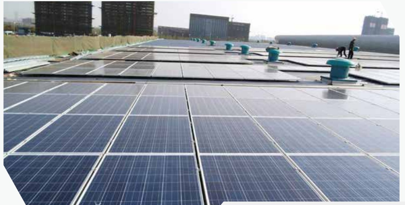
9.5MW power station on the roof of Hitachi Station
