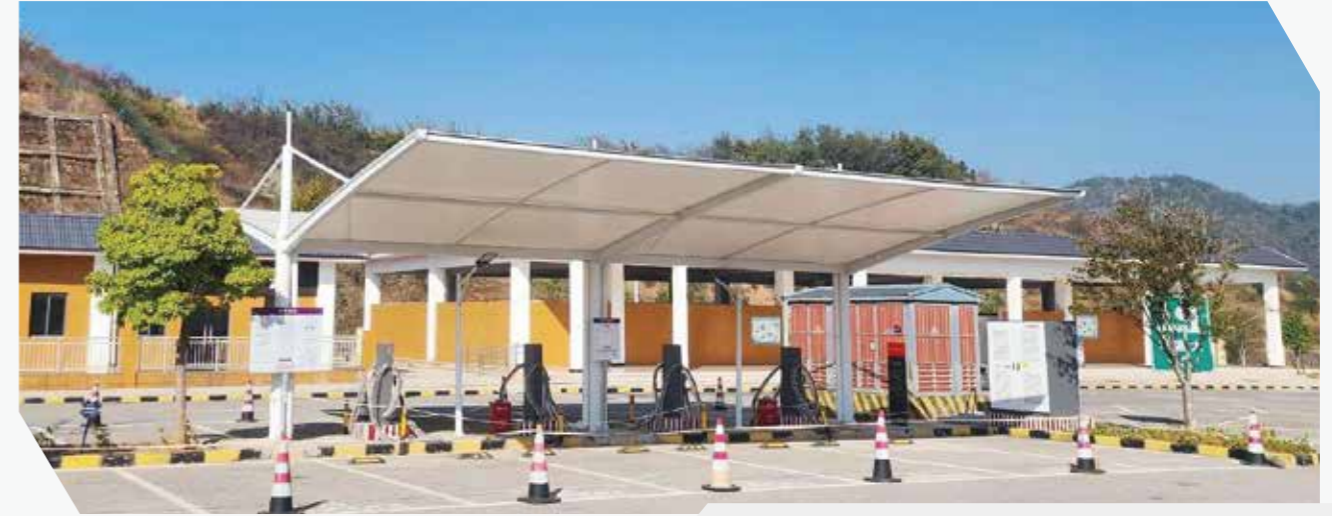
Bus optical storage charging power station project
