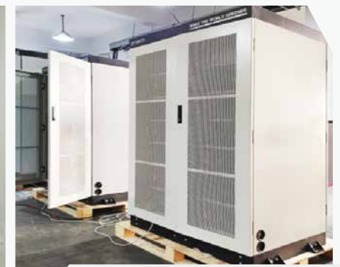
Botswana energy storage system project
