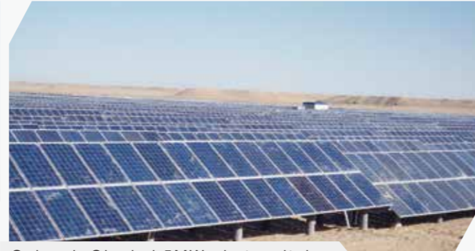
Golmud, Qinghai 5MW photovoltaic power station project
