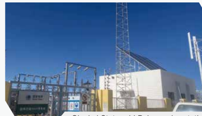
Qinghai State grid Balong relay station wind-wind complementary project
