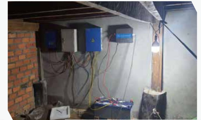
Cambodia 4kW-2kVA hybrid system
