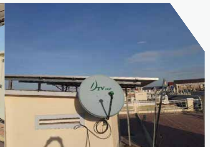
5 kW Off-Grid Solar System in Cambodia
