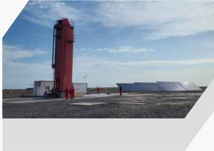
Microgrid System for Oil Extraction in Xinjiang, China
