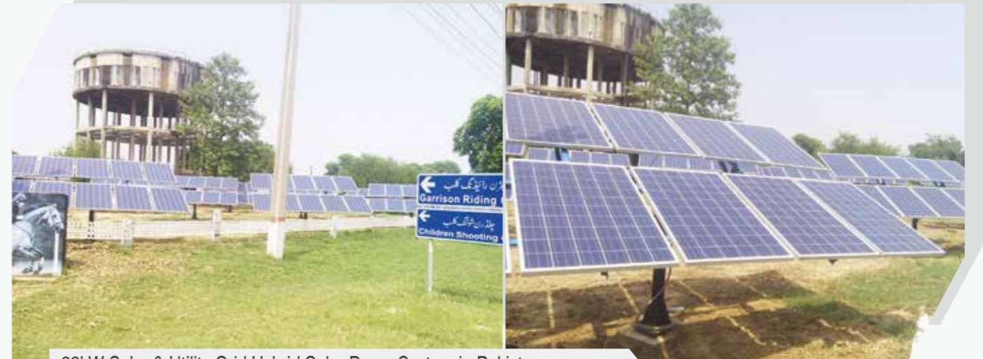
22kW Solar & Utility Grid Hybrid Solar Pump System in Pakistan
