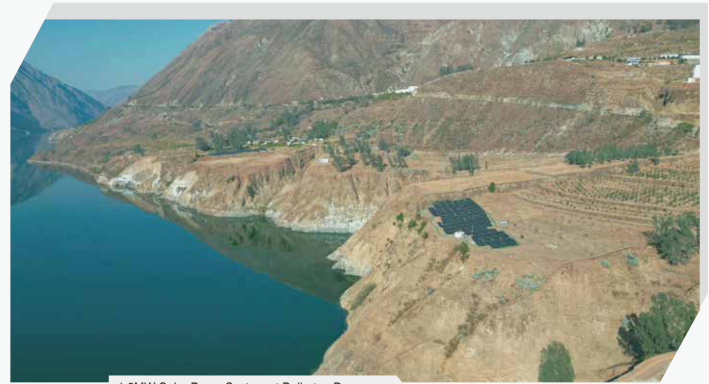
1.2MW Solar Pump System at Baihetan Dam
