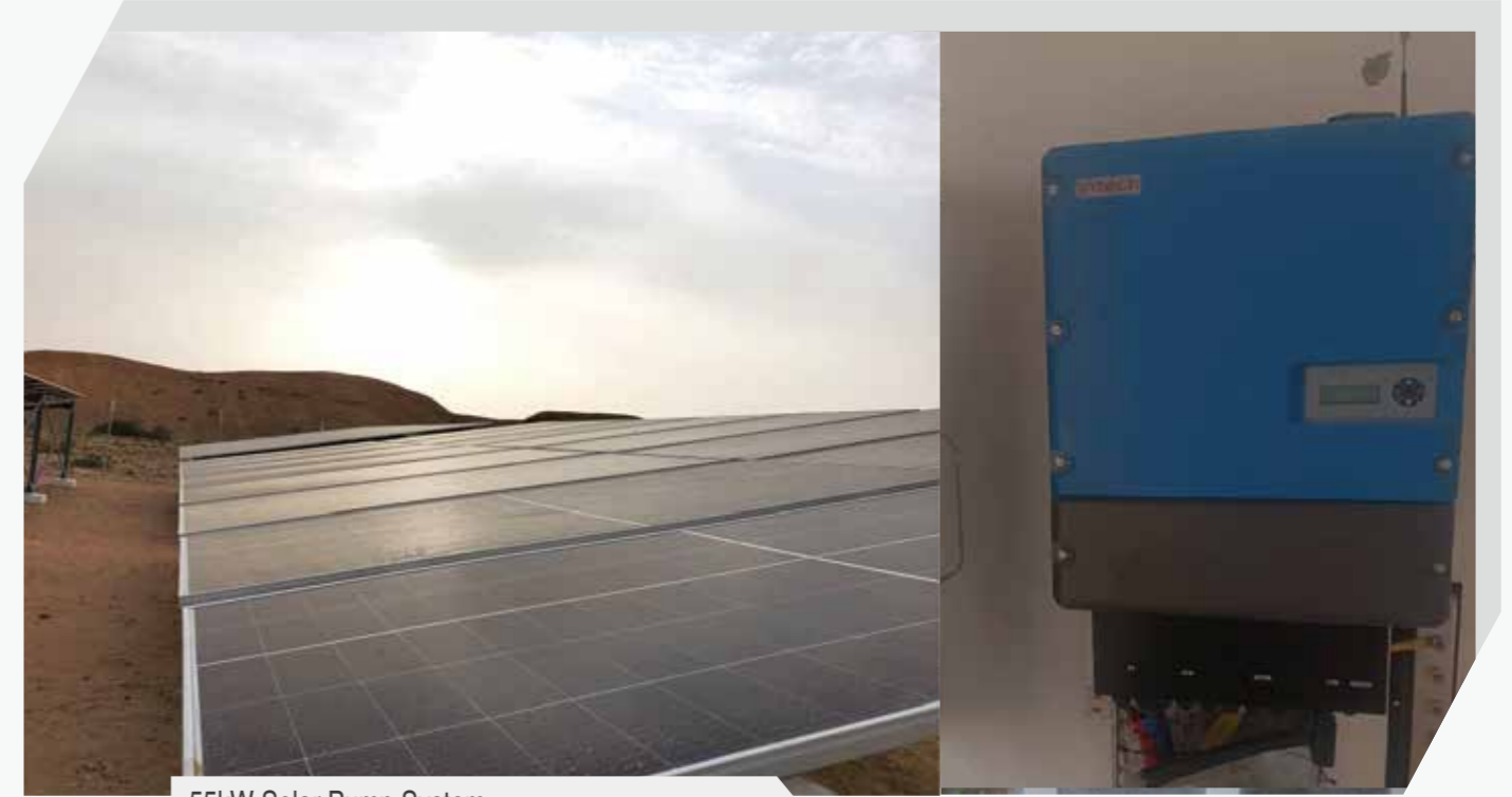
55kW Solar Pump System
