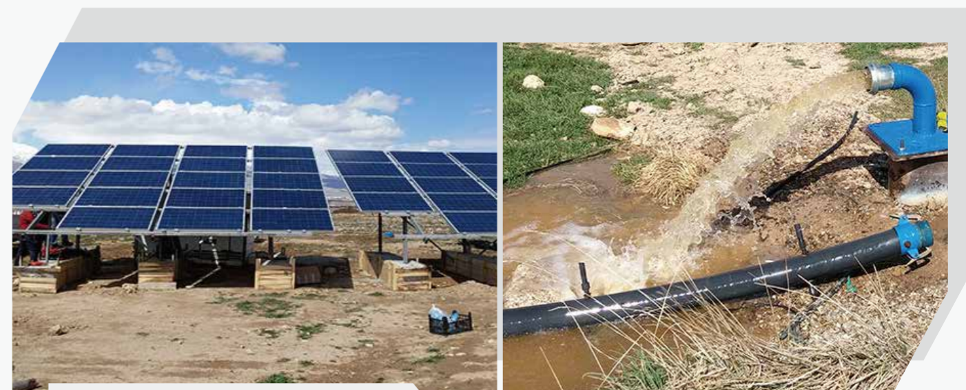
7.5kW Solar Pump System in Turkey
